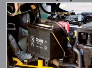
Rotational battery installation
